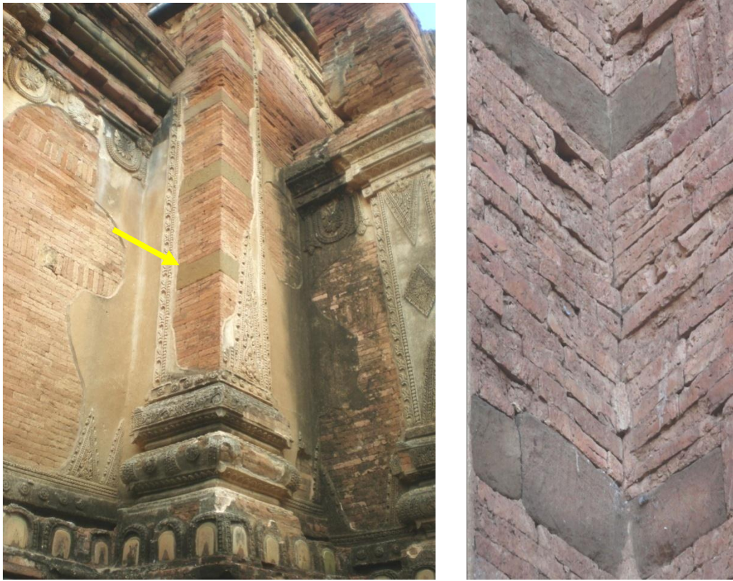
Fig-4, Right-angular shape reinforcement sandstone blocks from the corners of the main-body
