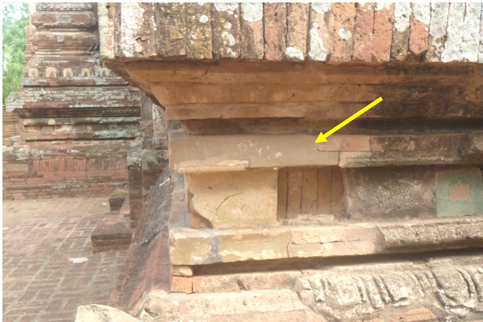
Fig-3, Reinforcement sandstone block at the corner of the brick laid above the recesses
